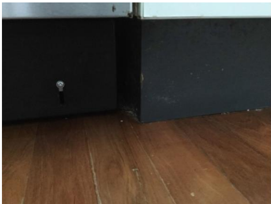
Water damaged floor
